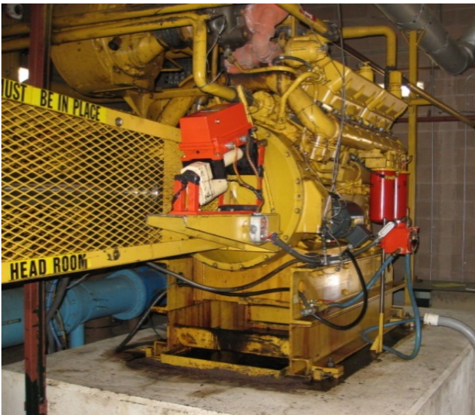
Corrales Well 5 Gas Engine
