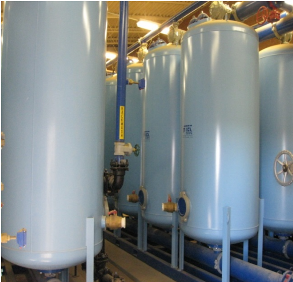
Corrales Well 3 - Arsenic Treatment System
