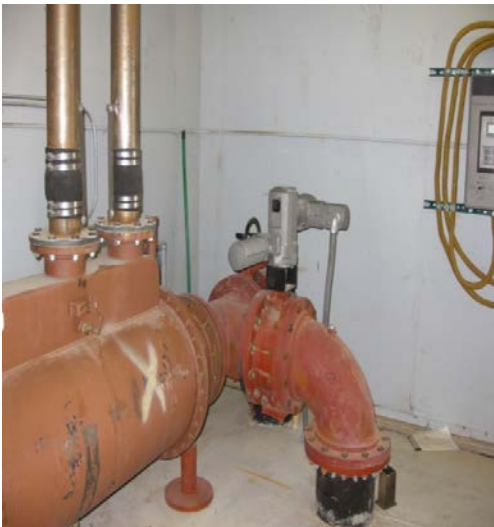
Corrales Well 2 Motorized Wash Line Valve Needs to be done at Corrales Well 8
