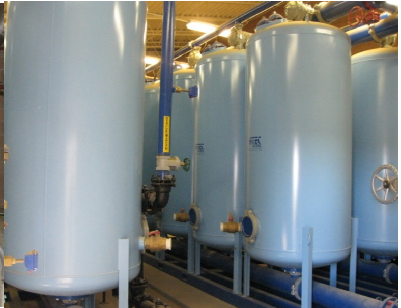
Arsenic Treatment Vessels
