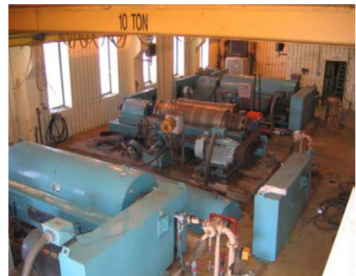
Centrifuge Room at existing SDF
