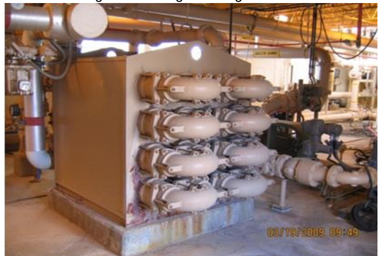
Digester Heat Exchanger for heating the sludge
