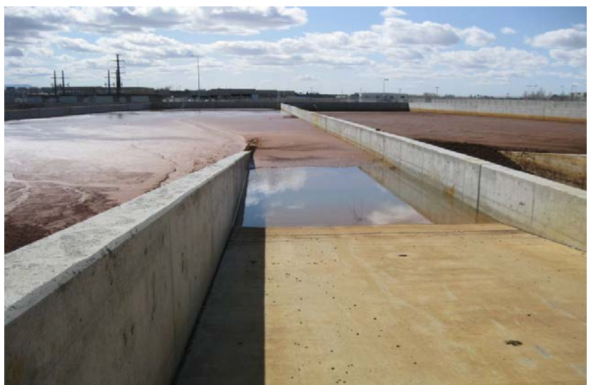
Ramp of Sludge Drying Bed at SJCWTP
