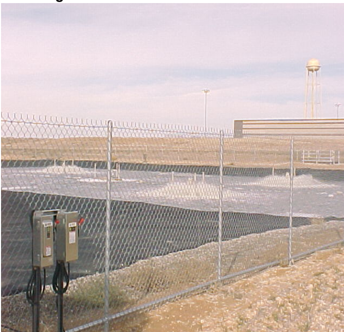
MDC Lagoon with Mixers and Aerators
