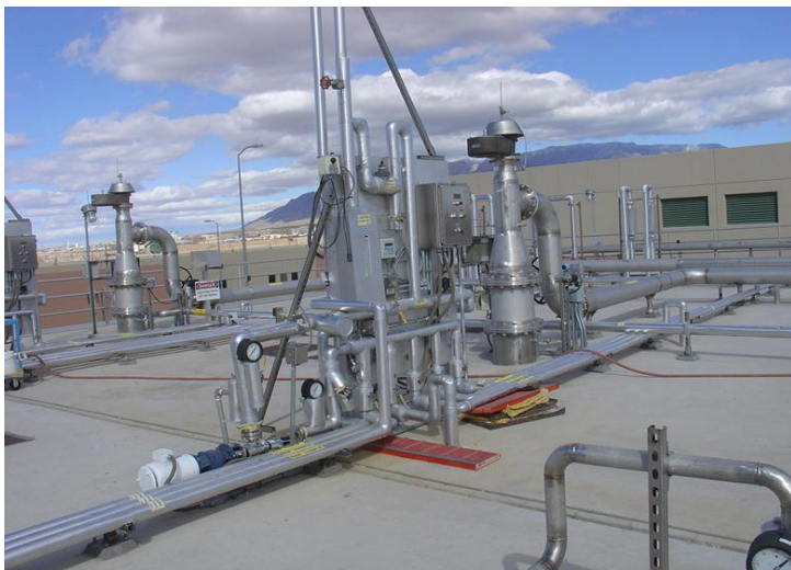
Ozone Monitoring Station Over Ozone Contactor Basins
