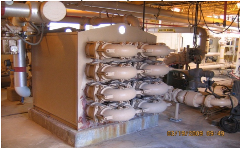
Digester Heat Exchanger for heating the sludge
