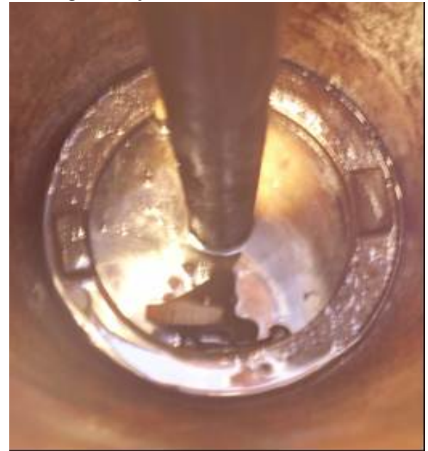
Leaking Fire Hydrant
