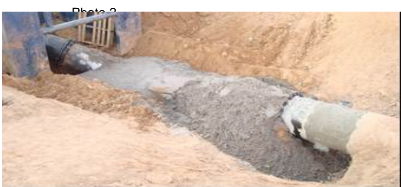
24" Concrete Cylinder Water Line Lowering and Relocation for a City Storm Drain Project in San Mateo NE
