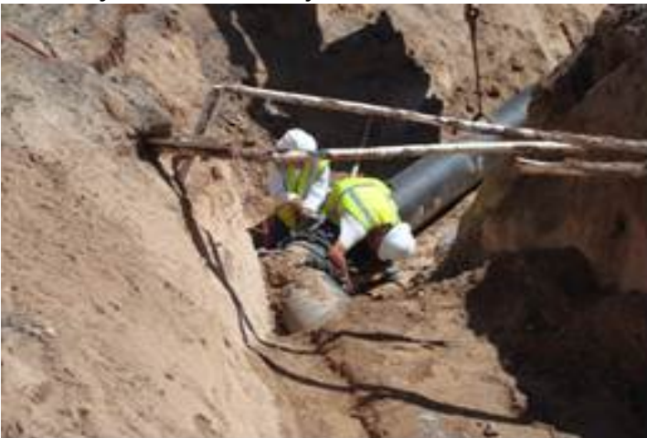
16" Ductile Iron Water Line Relocation for a City Storm Drain Project in Atrisco SW
