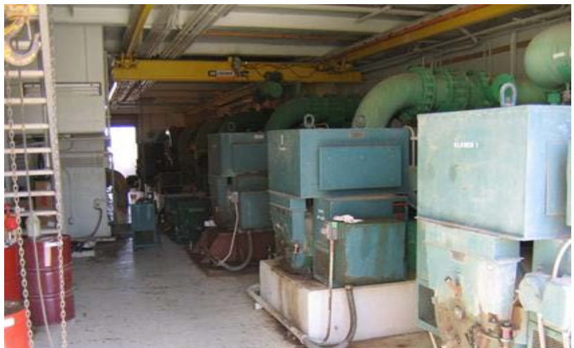
Aeration Basins Blowers
