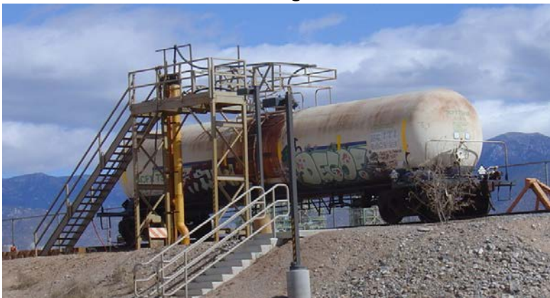
Ferric Chloride Railcar Unloading Station
