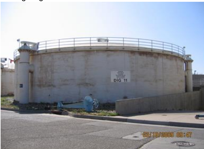
Existign digester at the SWRP
