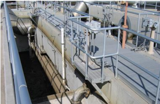
Aeration Tank Air Control Valve
