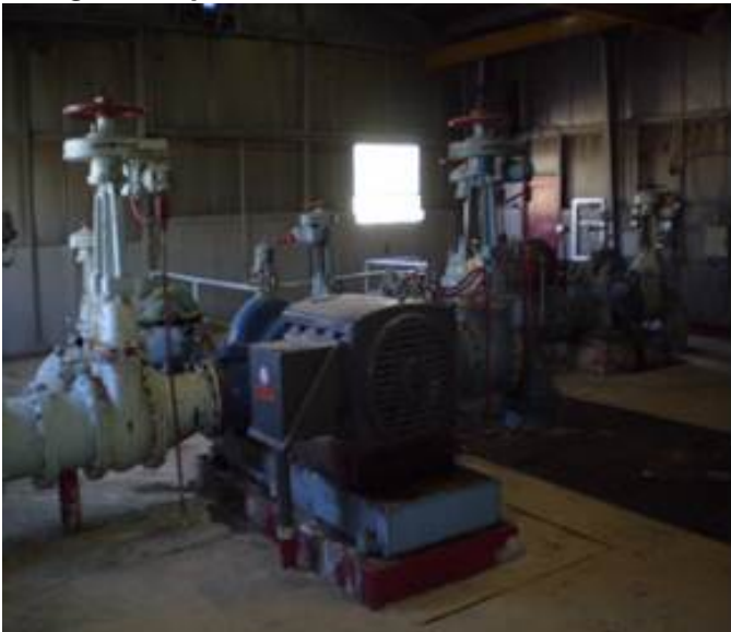
Griegos Pump Station - Interior
