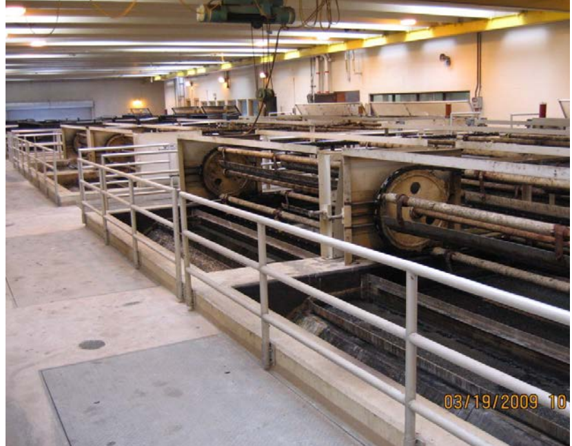
Looking North at the DAF tanks
