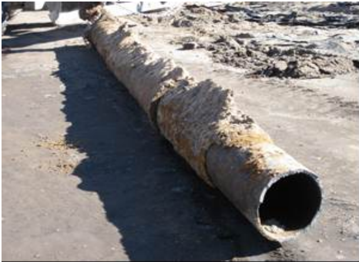
Corroded Steel Pipe
