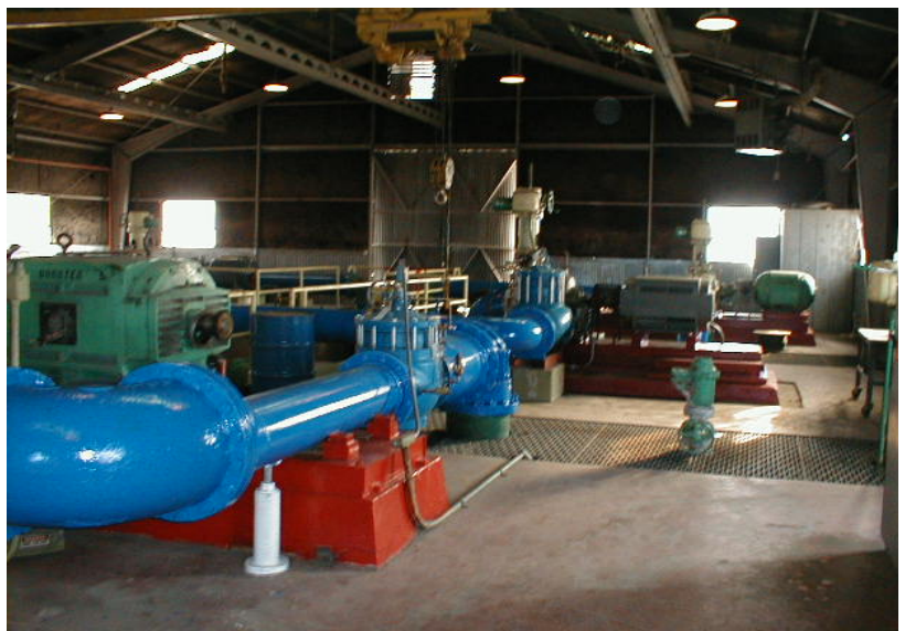
Santa Barbara Pump Station - Abandoned
