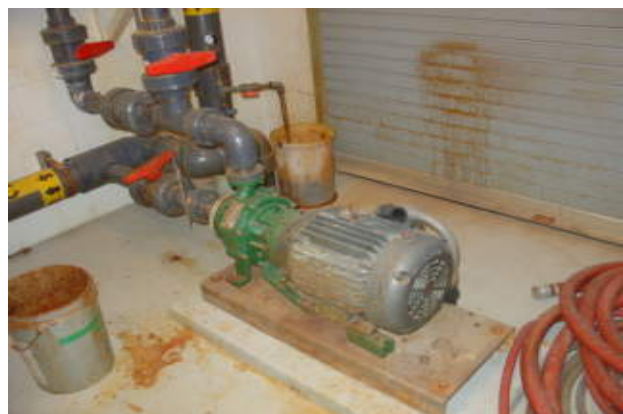
Ferric Chloride Transfer Pump
