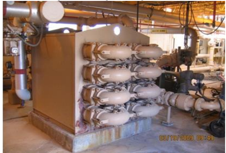
Digester Heat Exchanger for heating the sludge
