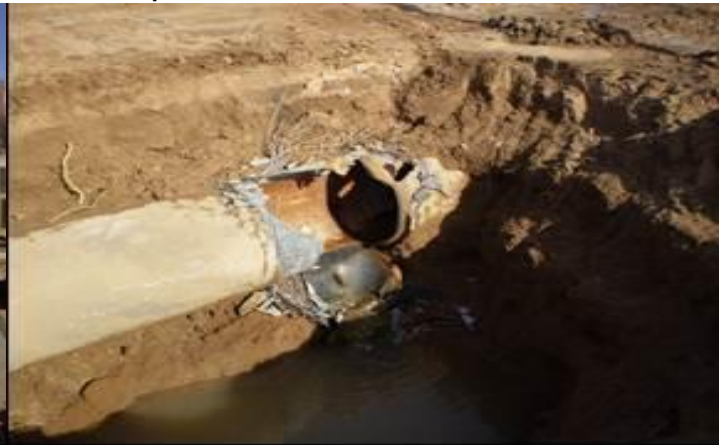
Valve to be replaced
