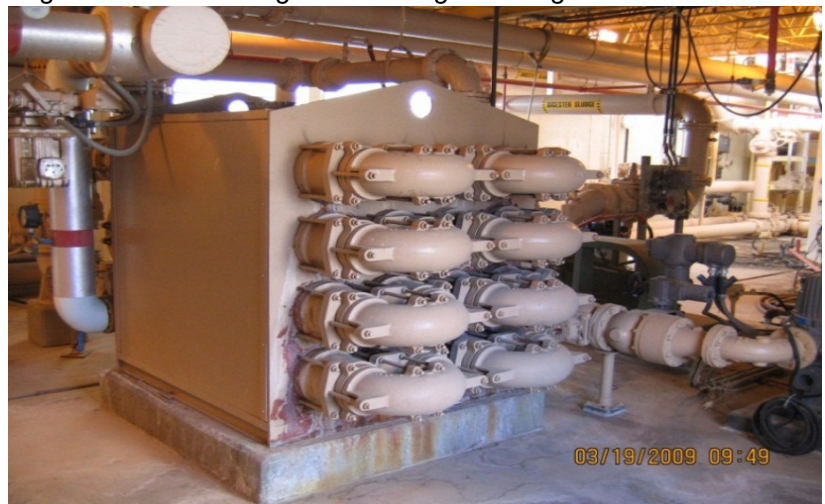
Digester Heat Exchanger for heating the sludge
