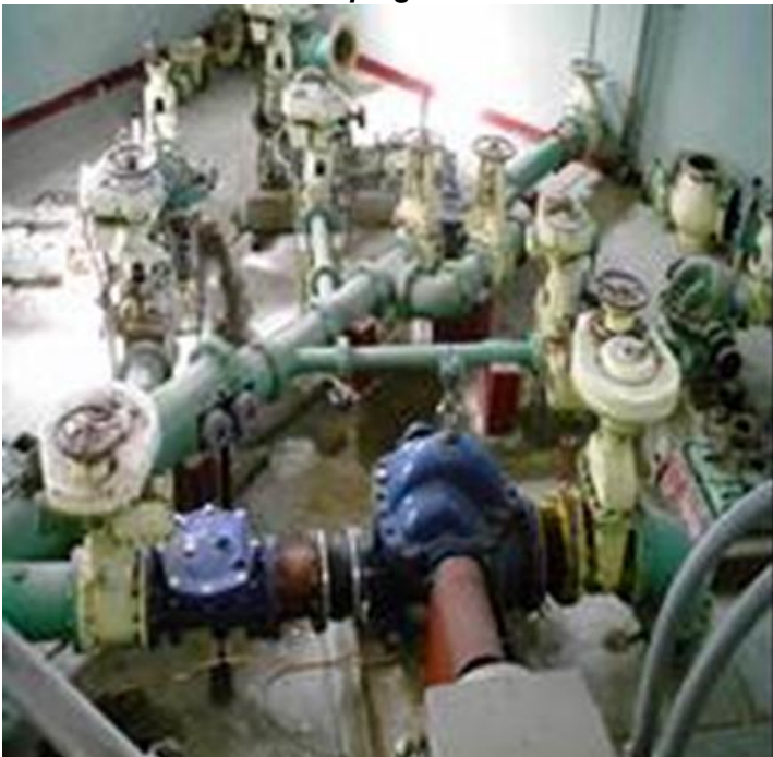
West Mesa Booster Pumping Station
