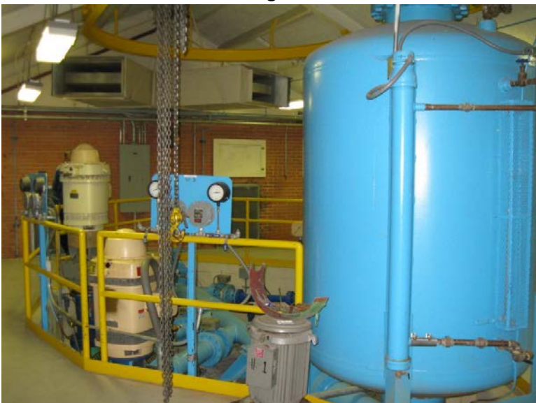
Canada Booster Station - Surge Tank
