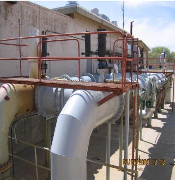
Lift Station #20 Force Main Header
