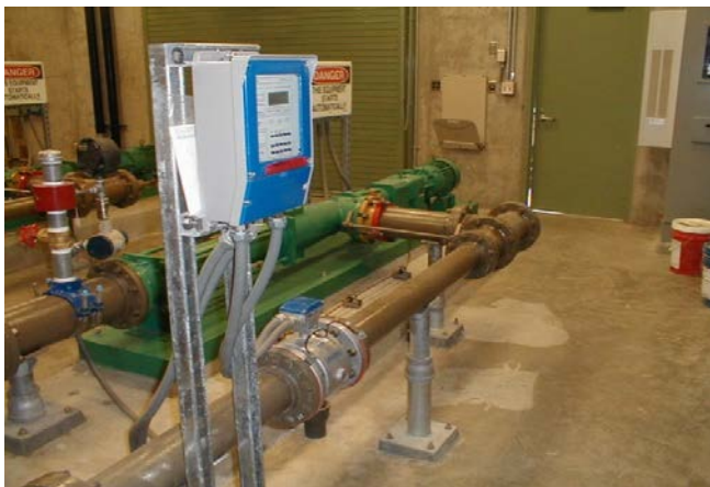
Progressive Cavity Sludge Pump at the WTP
