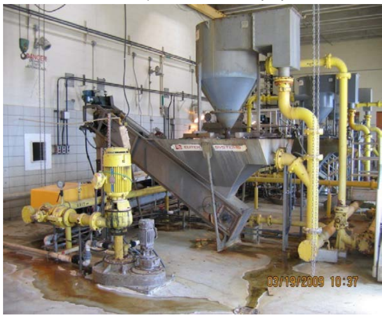
PTF Pista Grit Pump and Grit Recovery System
