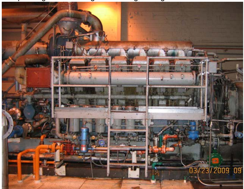
Cooper Cogeneration Engine at S.Cogen Bldg
