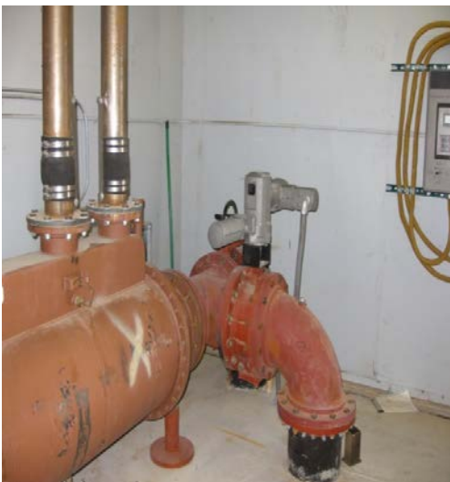
Corrales Well 2 Motorized Wash Line Valve Needs to be done at Corrales Well 9
