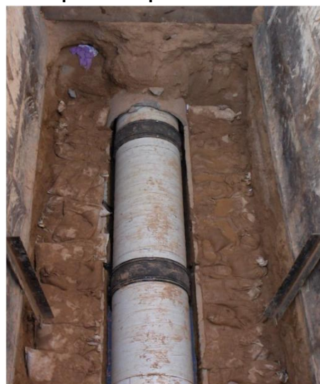
New 27-inch Sewer Line Sliplined in the old 30" Concrete Pipe in Prospect NE west of Carlisle
