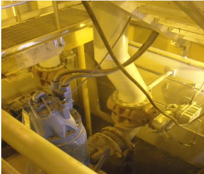
Lift Station #20 Pump & Piping
