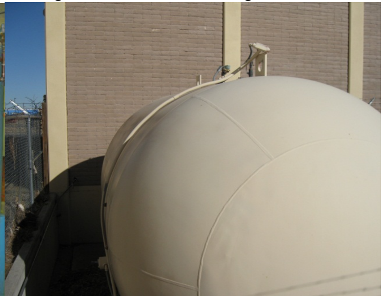
Ridgecrest Booster Station - Surge Tank
