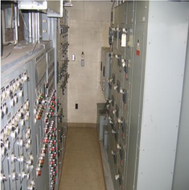
Typical MCC Switchgear
