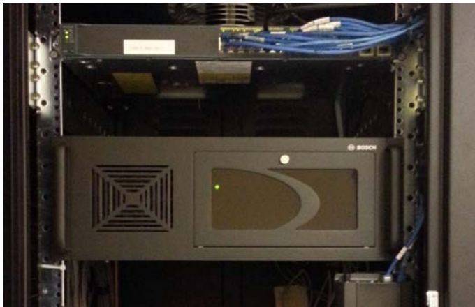
Computer components are obsolete
