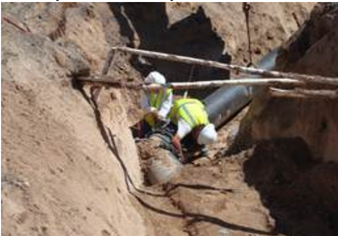
16" Ductile Iron Water Line Relocation for a City Storm Drain Project in Atrisco SW
