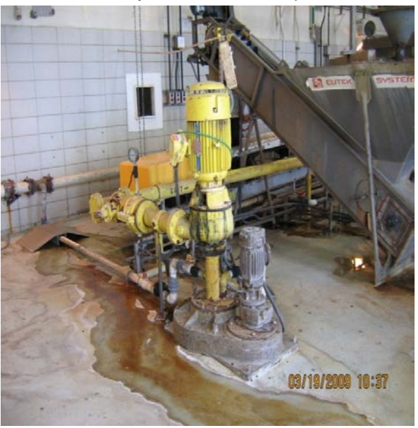
PTF Pista Grit System Grit Lift Pump
