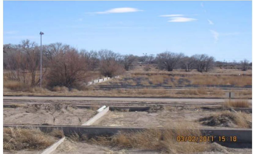
Sludge Drying Beds that were added in 1980's
