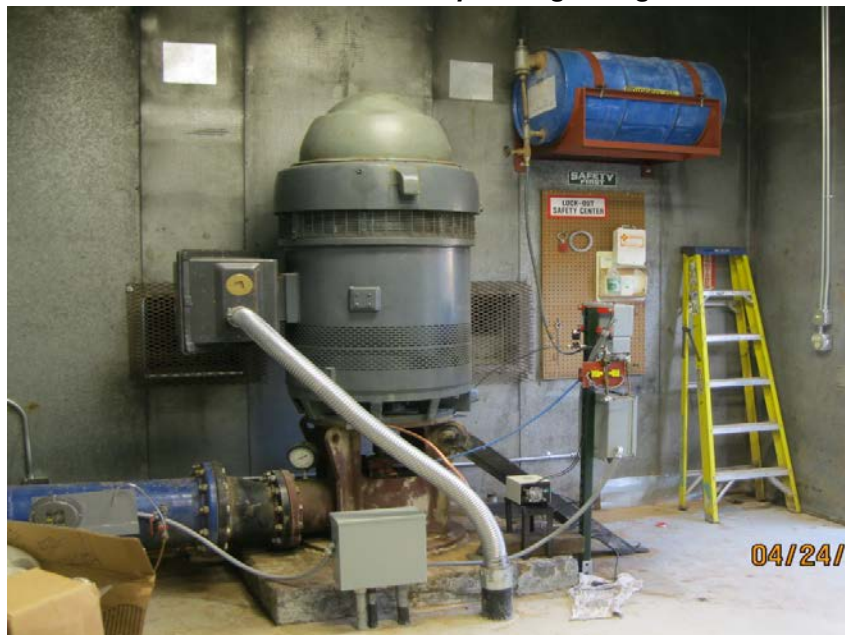
Corrales Well 1 - Electric driver replaced gas engine
