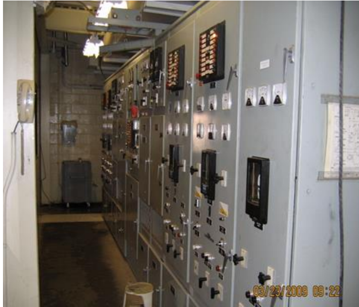
South Cogen Switchgear
