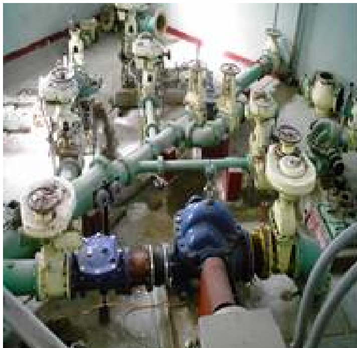
West Mesa Booster Station
