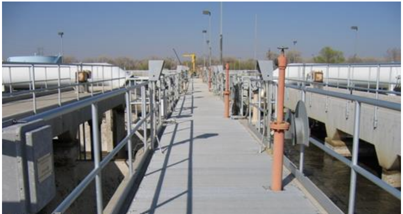
Aeration Tanks catwalk
