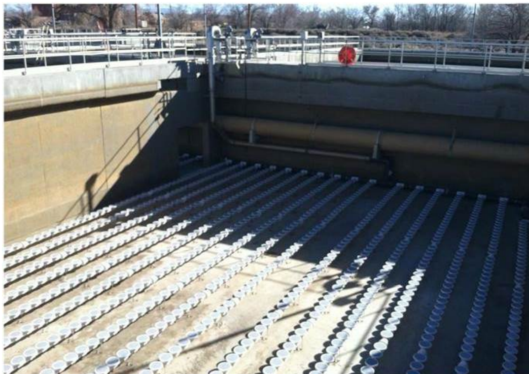
Aeration Basin with Air Diffusers on the Bottom
