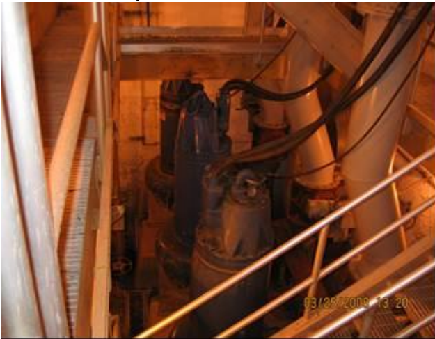
Lift Station Pumps
