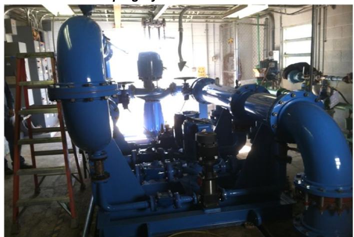
SAF Water Pumping System
