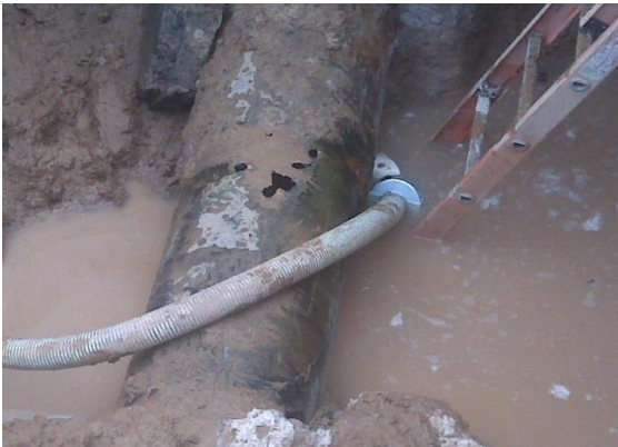
Hole in 20" Diameter Steel Water Line
