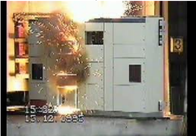
Arc flash at an electrical panel
