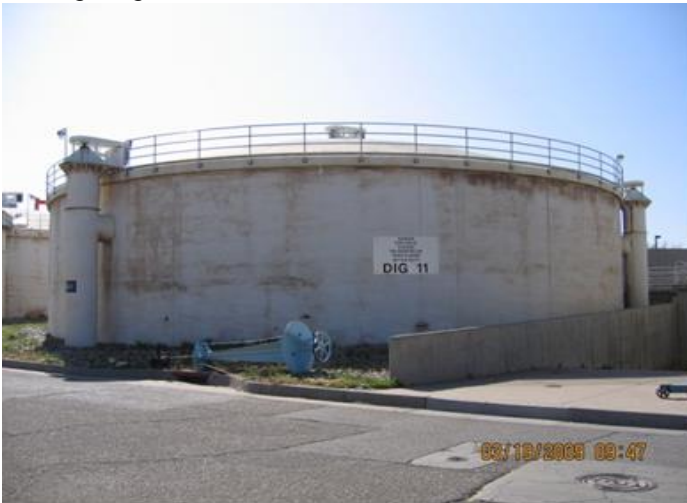
Existign digester at the SWRP
