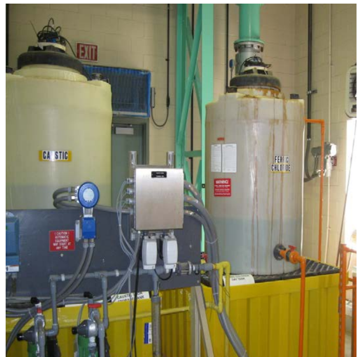
Chemical Feed Systems
