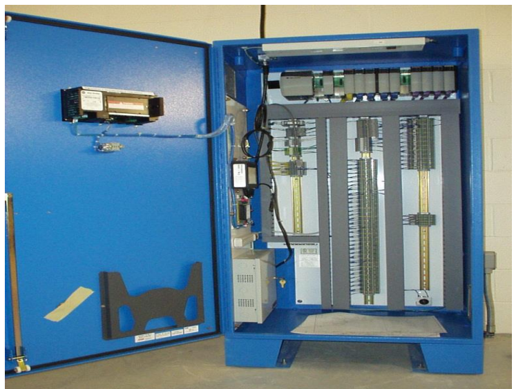
Typical ControlLogix PLC
