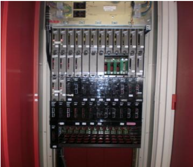
ABB Process Control Unit
