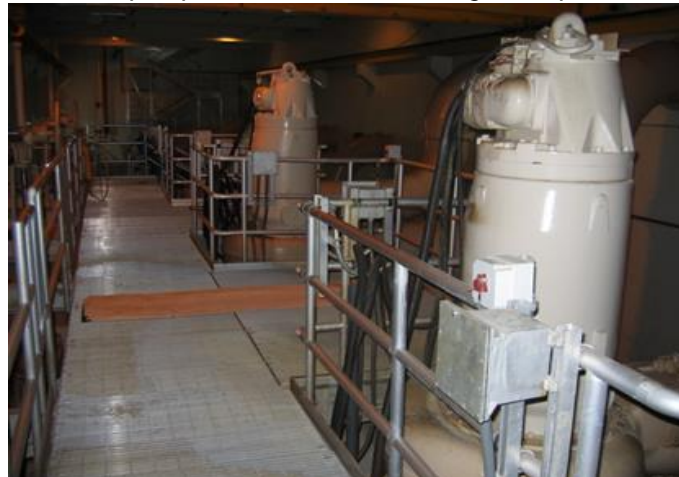
View of RAS pumps inside Activated Sludge Pump Sta
