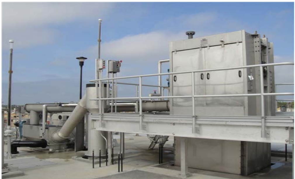
Band screen installation with screenings conveyance
