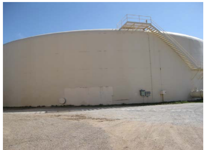
Coronado Reservoir - Steel Tank
