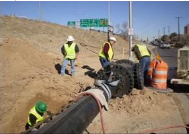
Large Valve, east of I-25
