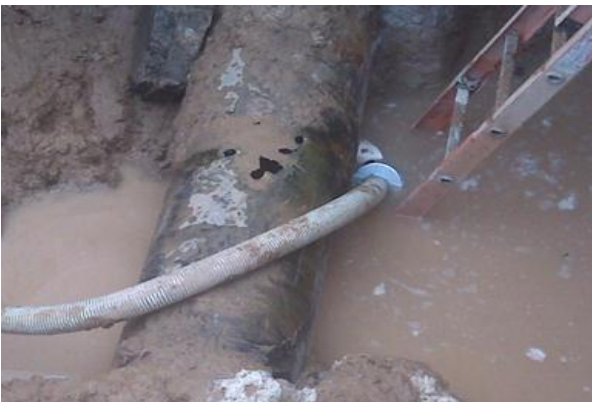
Holes in a 20-inch Water Line
