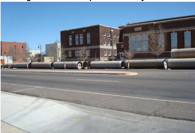
New 48" Sewer Line to be Slip-lined into an existing 54" Concrete Pipe in Broadway NE
