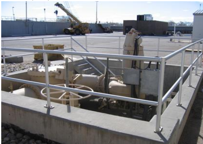
4th RAS pump which is installed outdoors
