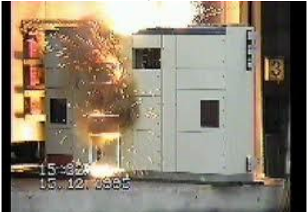
Arc flash at an electrical panel
