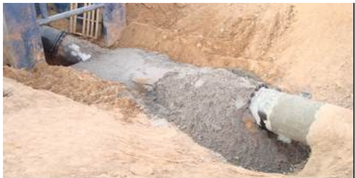
24" Concrete Cylinder Water Line Lowering and Relocation for a City Storm Drain Project in San Mateo NE
