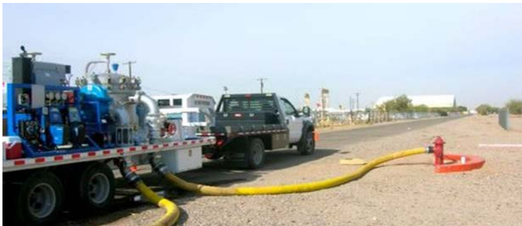
Water Line Flushing Filtration Unit
